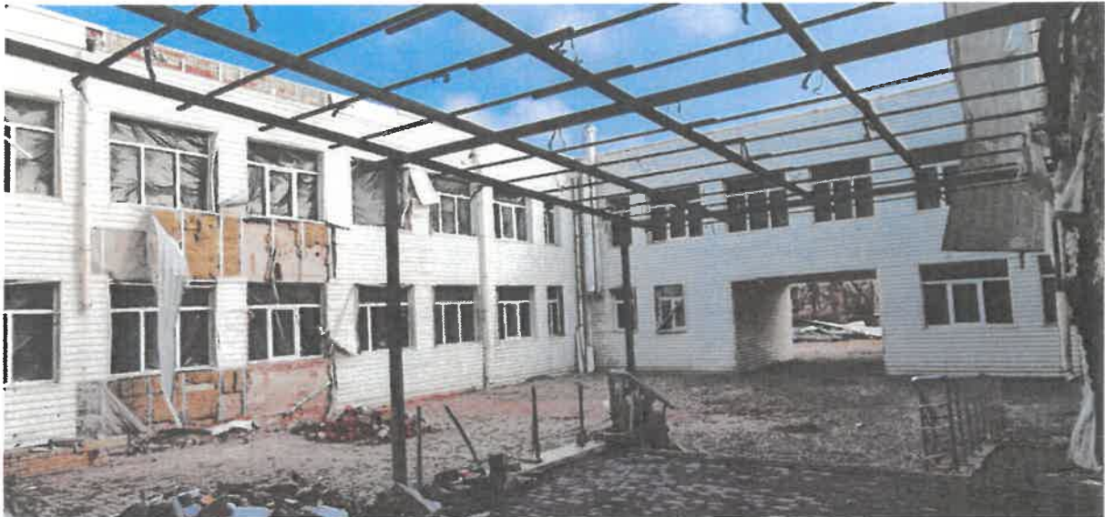
Bombed school in Korobochkyne
